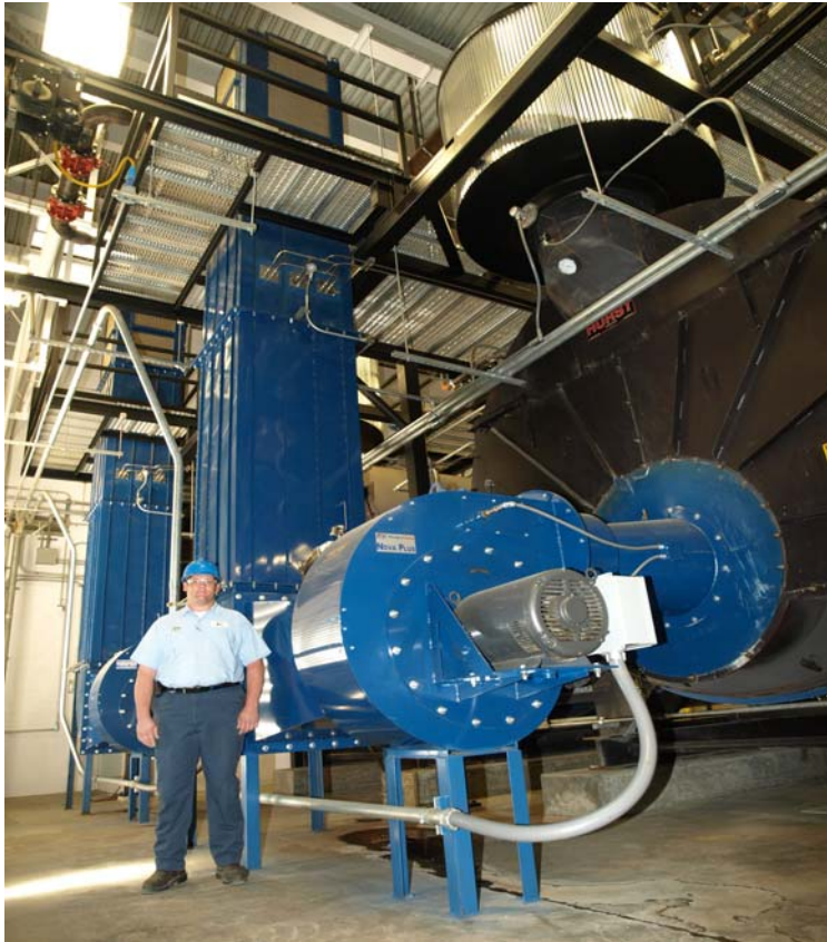
Mike Alles – Facilities Superintendent in front of the LNINVC17 burners & Hurst Boilers
